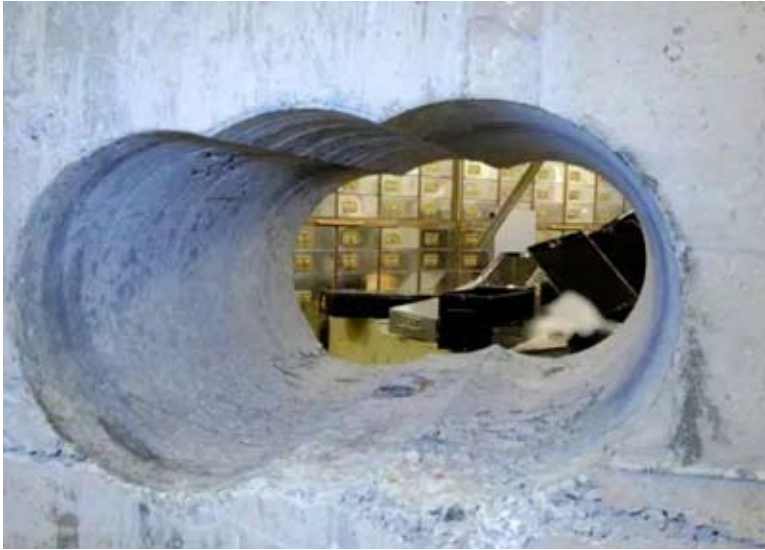
Holes bored through a half-metre thick concrete wall to access a vault in a safe deposit centre in Hatton Garden, London, where £14 million of diamonds and jewellery were stolen between April 2 and April 5, 2015.
